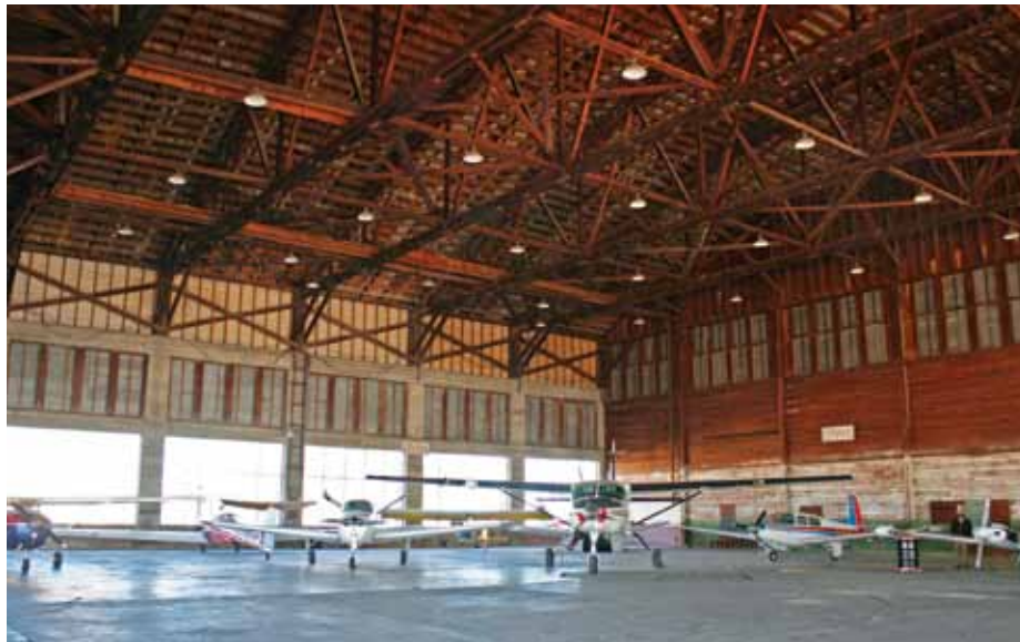
Above, Great Bend air field hangar, Barton County; Below, Great Bend Norden Bombsight Storage Vaults, Barton County.
